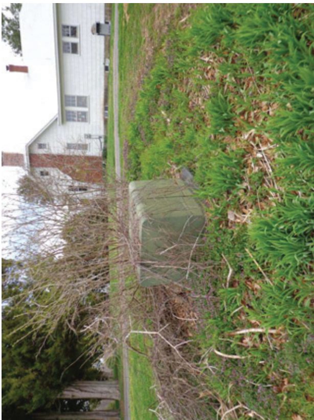
PHOTO 12: Pad-mounted Transformer (located east of residence)
